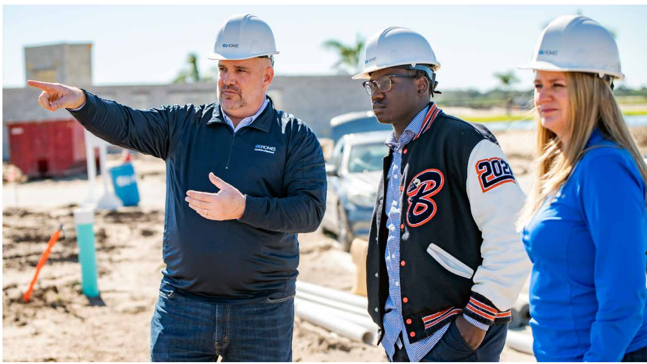
GL Homes Director of Land Development Anthony LoFurno and GL Homes Project Engineer Heather Swanson talk about the Valencia Grand project site with Boys & Girls Club member Kelvin Rolle, an aspiring civil engineer. TRACEY BENSON PHOTOGRAPHY
